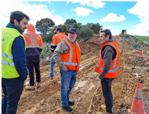
Photo: Pedro Serrano Dorado Head of Development GPG, Borja Franciso Valdes GPG Site Manager, Alfonso Monedero Llorente GPG C3 Assistant Dir. Weekly Site Inspection.
