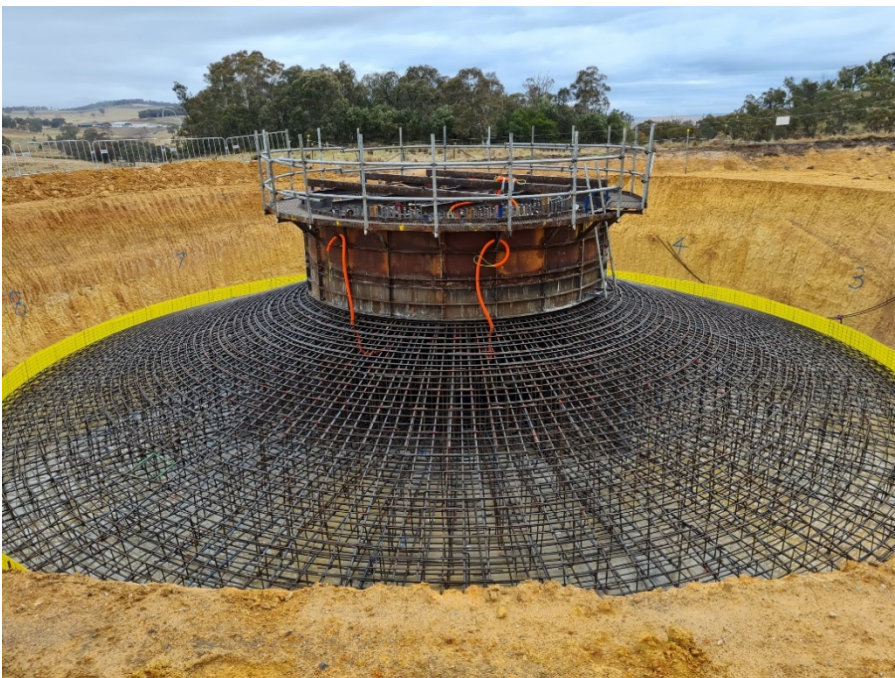
Foundation containing the anchor cage and steel structure ready to be concrete poured
