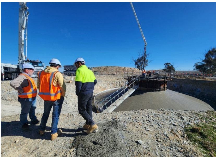
GPG team inspecting one of the foundations while concrete is being poured
