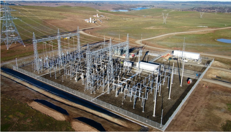
Substation which connects Crookwell 2 & 3 Wind Farms to the Grid
