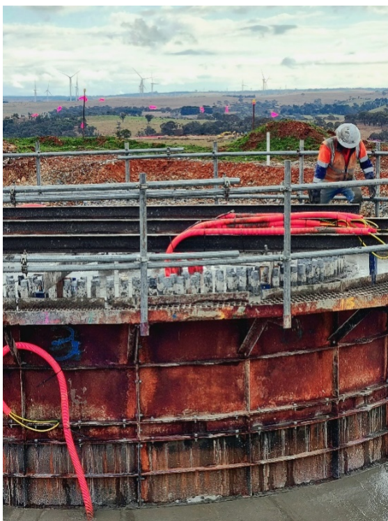
Tradesman working in one of the foundations at Crookwell 3, with the Crookwell 2 turbines on the horizon
