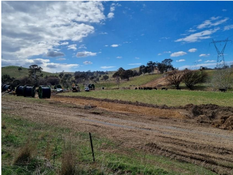
RJE Global is currently working on Woodhouselee Road on their way to the Substation located in Crookwell 2. Traffic management is in place.
