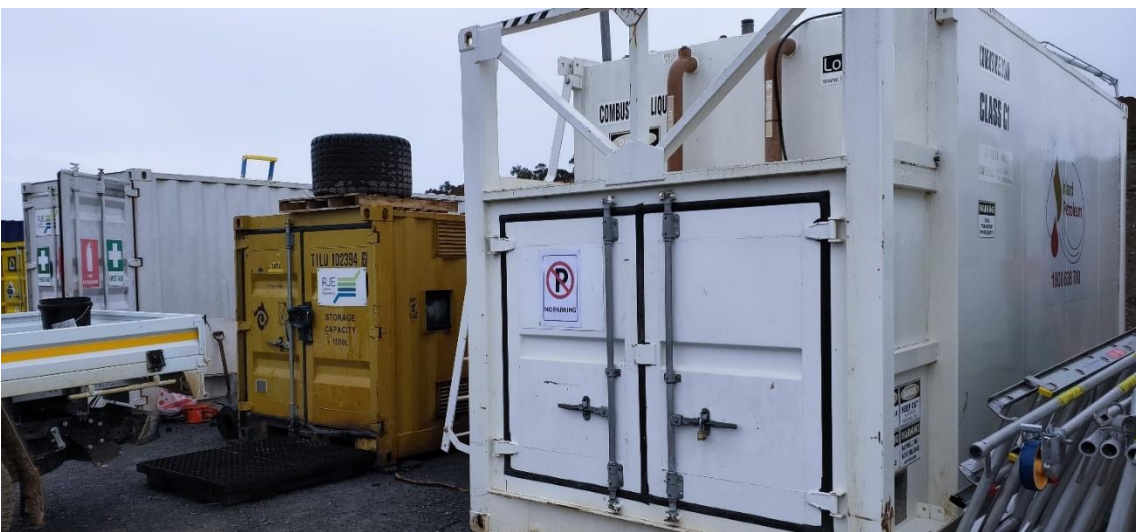
Photograph 8 – Chemicals correctly stored in self bunded tanks and with spill prevention
