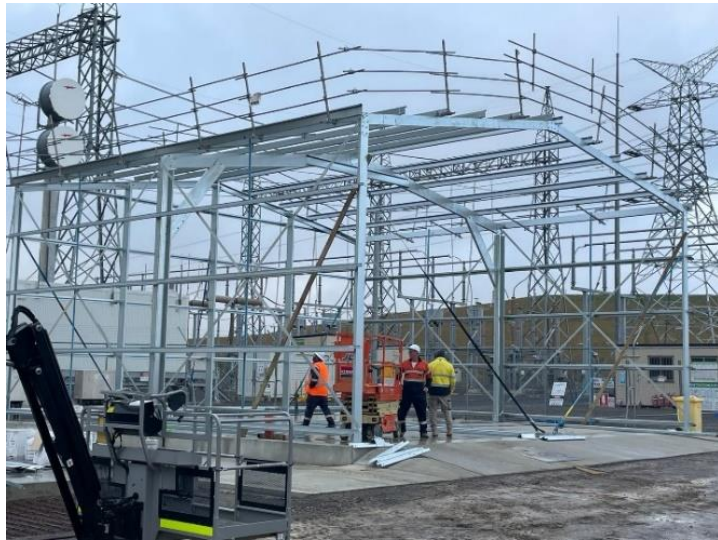
A warehouse is currently being built onsite at Crookwell 2 Wind Farm. It will have maintenance and repair equipment for both wind farms and will be shared by General Electric and Vestas.
