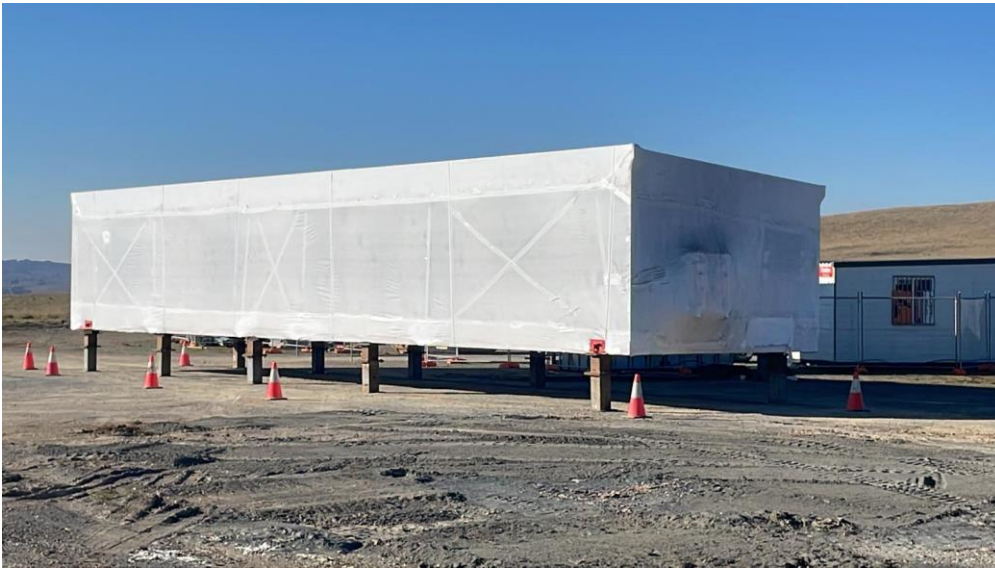
The first part of the substation building has been delivered at Crookwell 2 Wind Farm.
